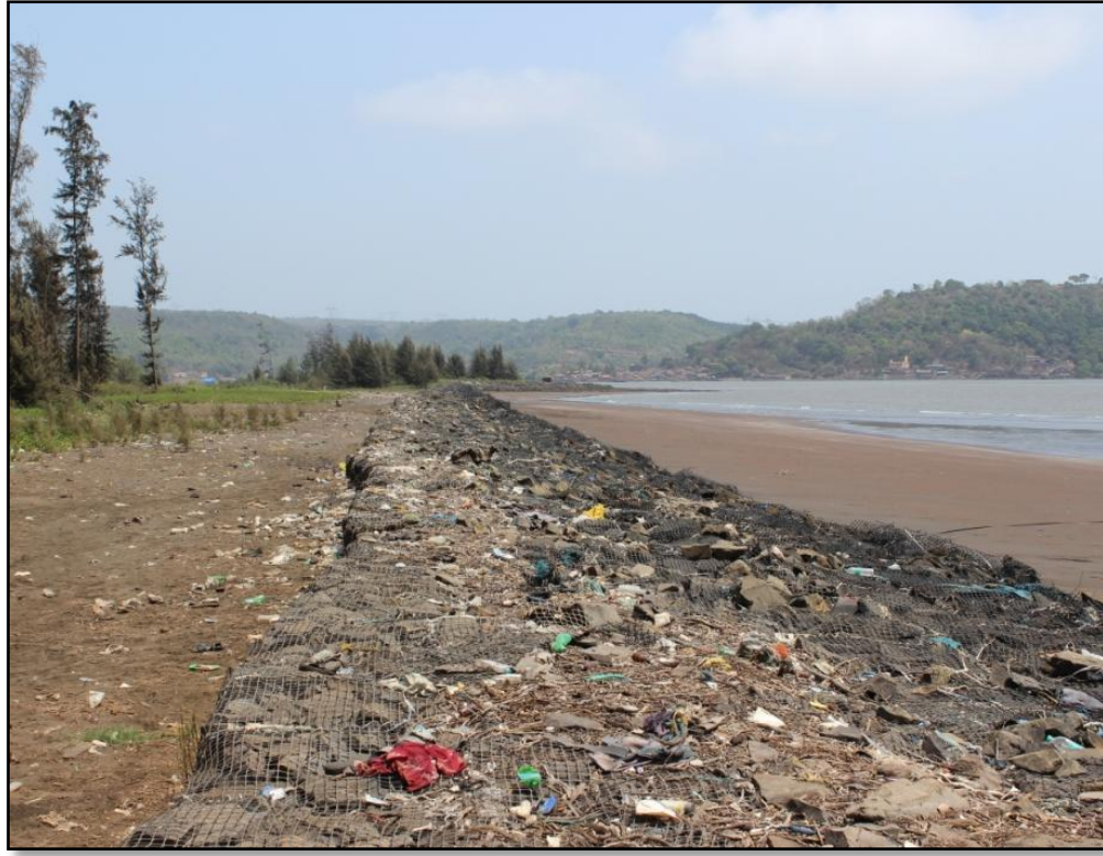
Plate 33: Coastal protection measures at the northern bank of Vashishti River mouth (47G02SE)
