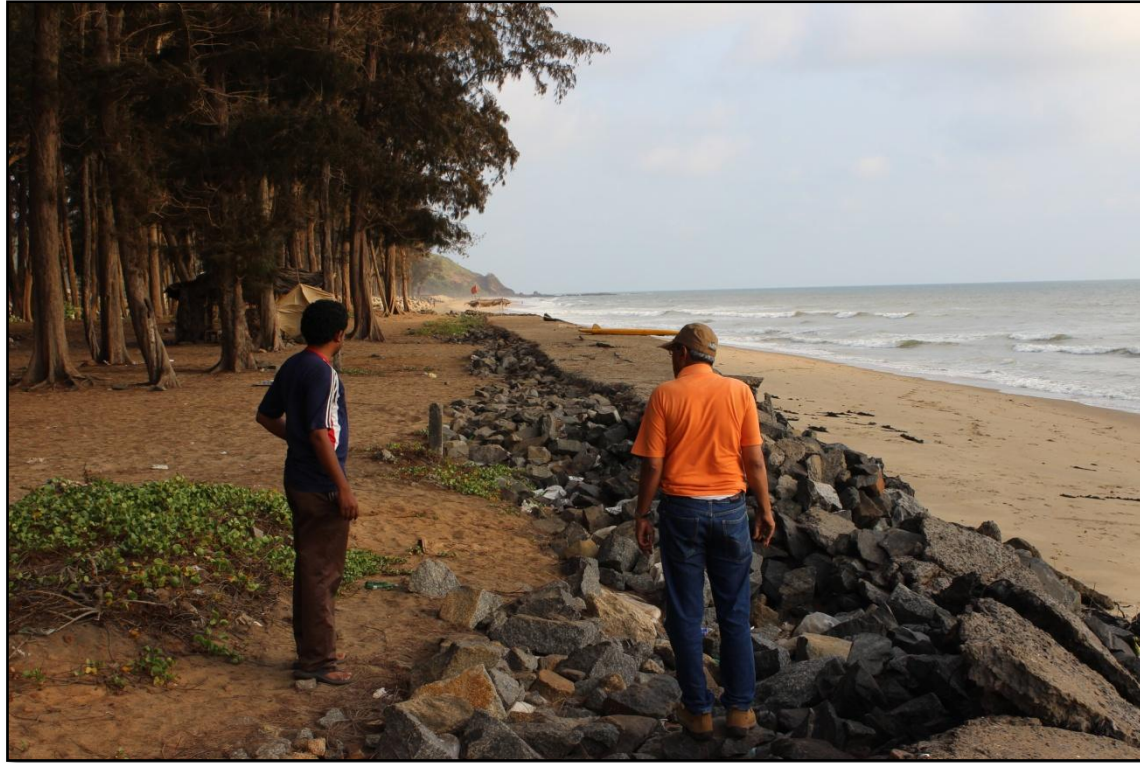
Plate 48: Damaged sea wall at Keri (46E10NE)
