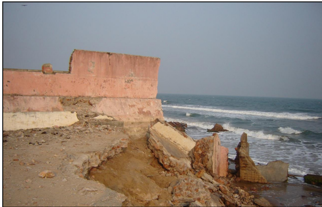
Plate 23: Hatcheries destroyed due to coastal erosion near Shamvanipakalu (65K08SE)
