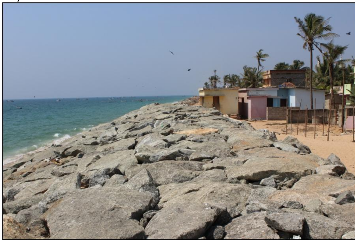
Plate 77: Sea wall at Puttantura, Kanniyakumari district (58H04NE)
