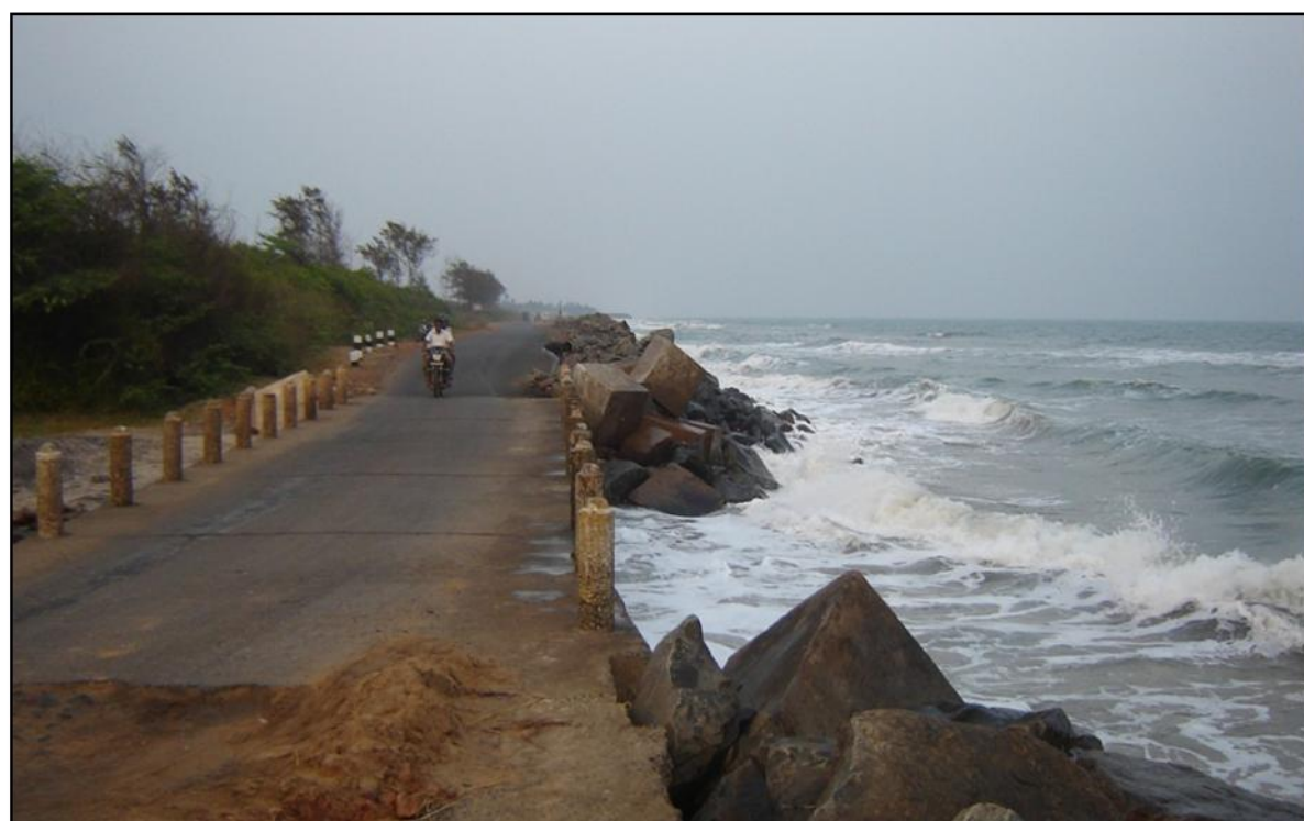
Plate 30: Road between Uppada – Kakinada marks the sea limit and is exposed to coastal erosion (65K08SW)
