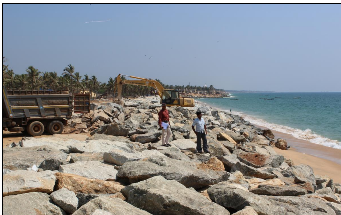
Plate 78: Sea wall at Puttantura, Kanniyakumari district (58H04NE)
