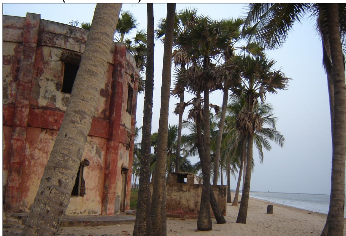
Plate 36: Severe erosion, west of Vasishta Godavari river mouth, sand dune ridge in front of cyclone shelter totally eroded (65H11SE)
