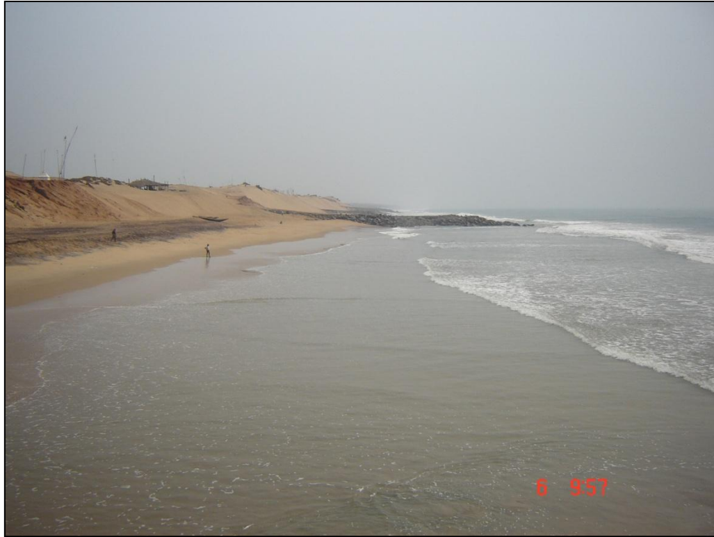
Plate 16: Groyne constructed for beach nourishment on northern parts of Old Gopalpur Port (74A15SE) on southern Odisha coast
