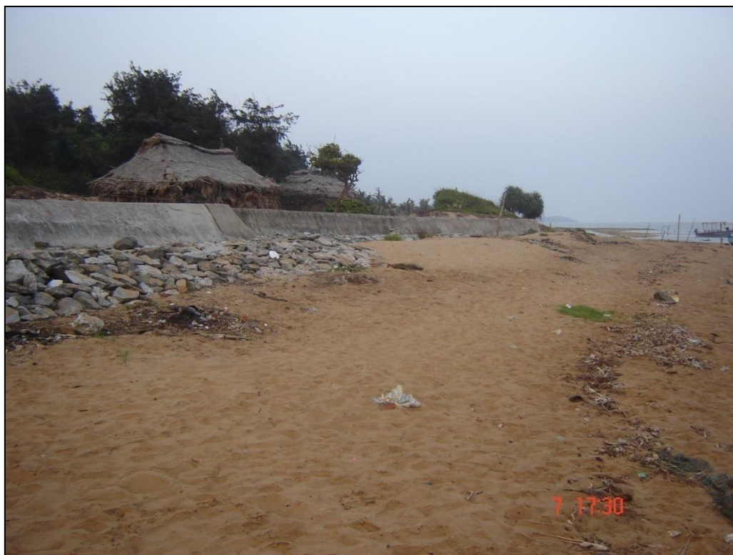
Plate 33: Sea wall/embankment on the eastern parts of the Kushabhadra river, near Maa Ramachandi temple, Puri district, Odisha (74IO1SW)
