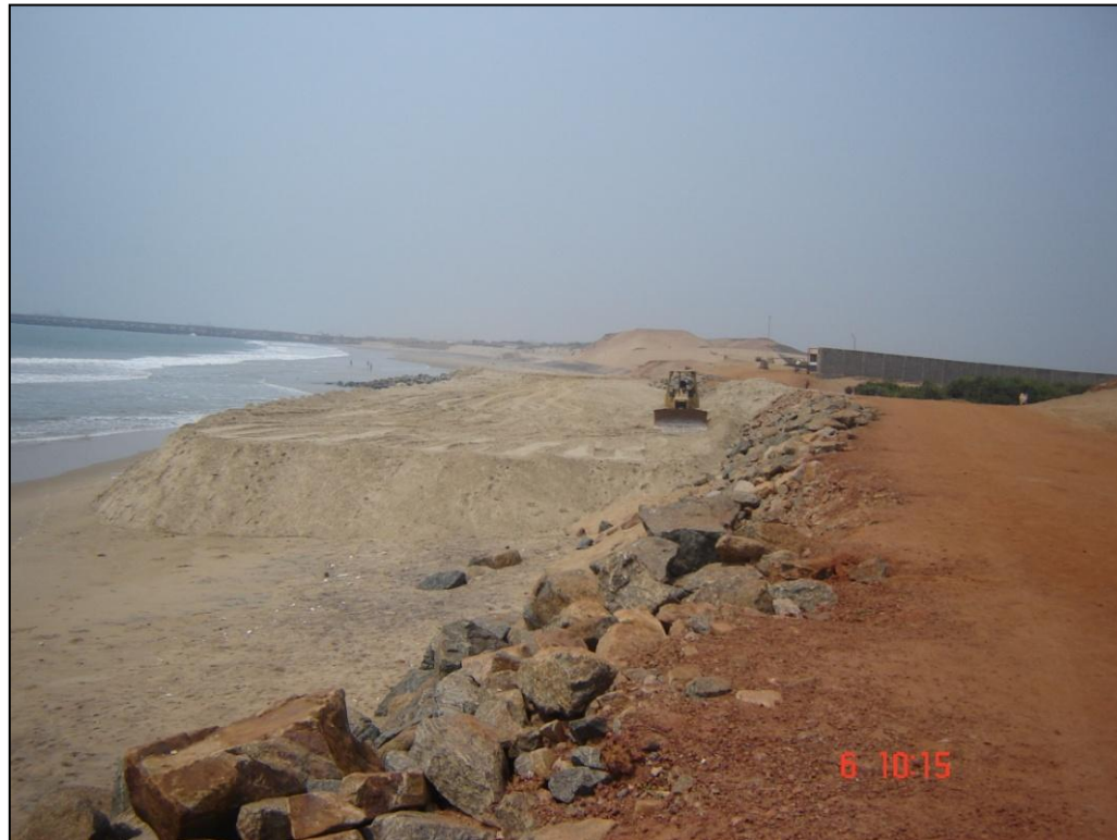
Plate 17: Groyne under construction for beach nourishment on northern parts of Old Gopalpur Port (74A15SE) on southern Odisha coast
