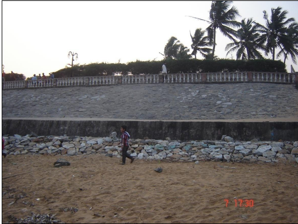
Plate 34: Sea wall/embankment on the eastern parts of the Kushabhadra river at Maa Ramachandi temple, Puri district, Odisha (74IO1SW)
