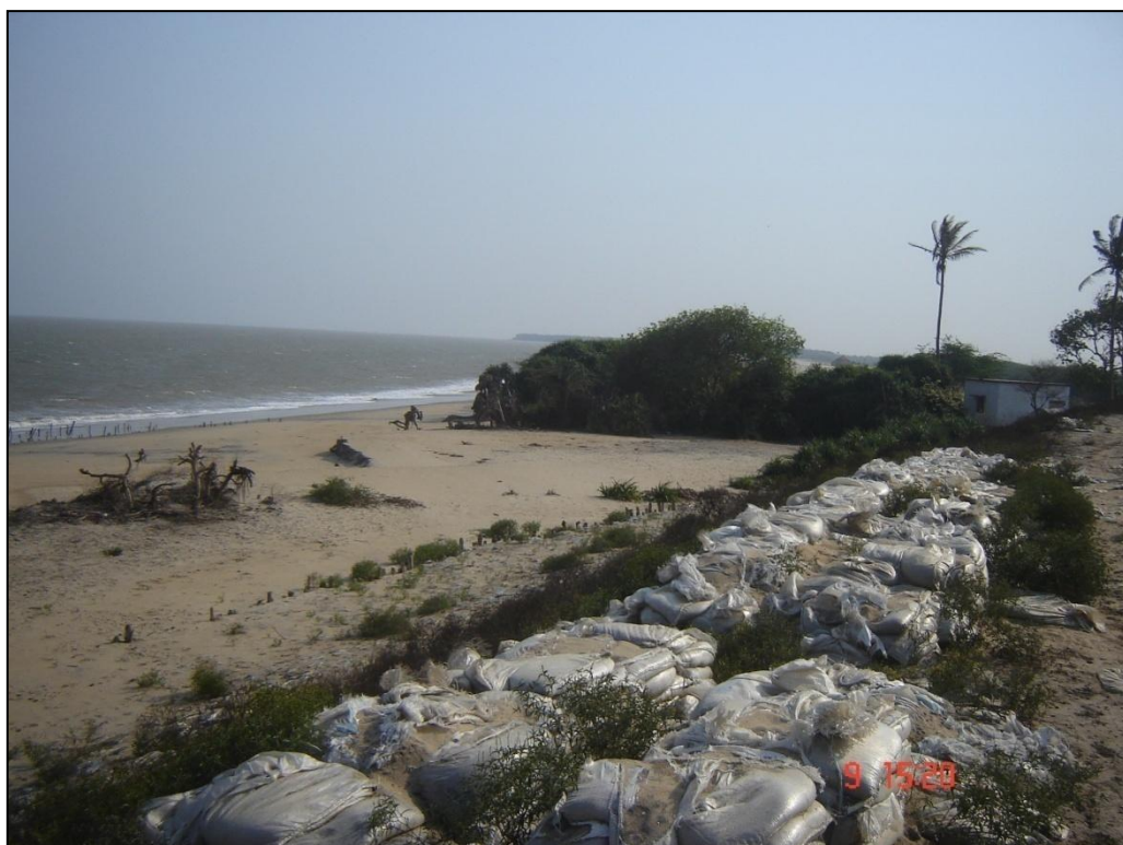
Plate 42: Protection of the embankment at Pentha (73L14SW) along central parts of Odisha coast
